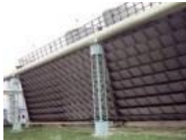
Cooling tower blowdowns
