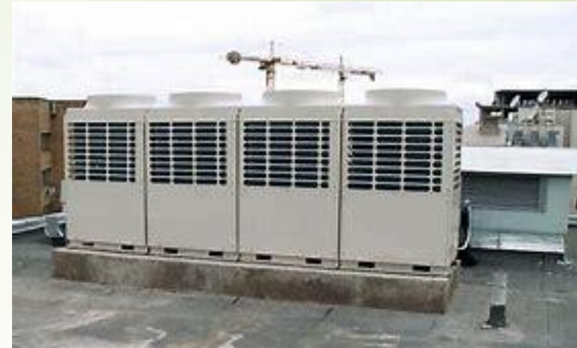
Hot Air Exhaust Vent
